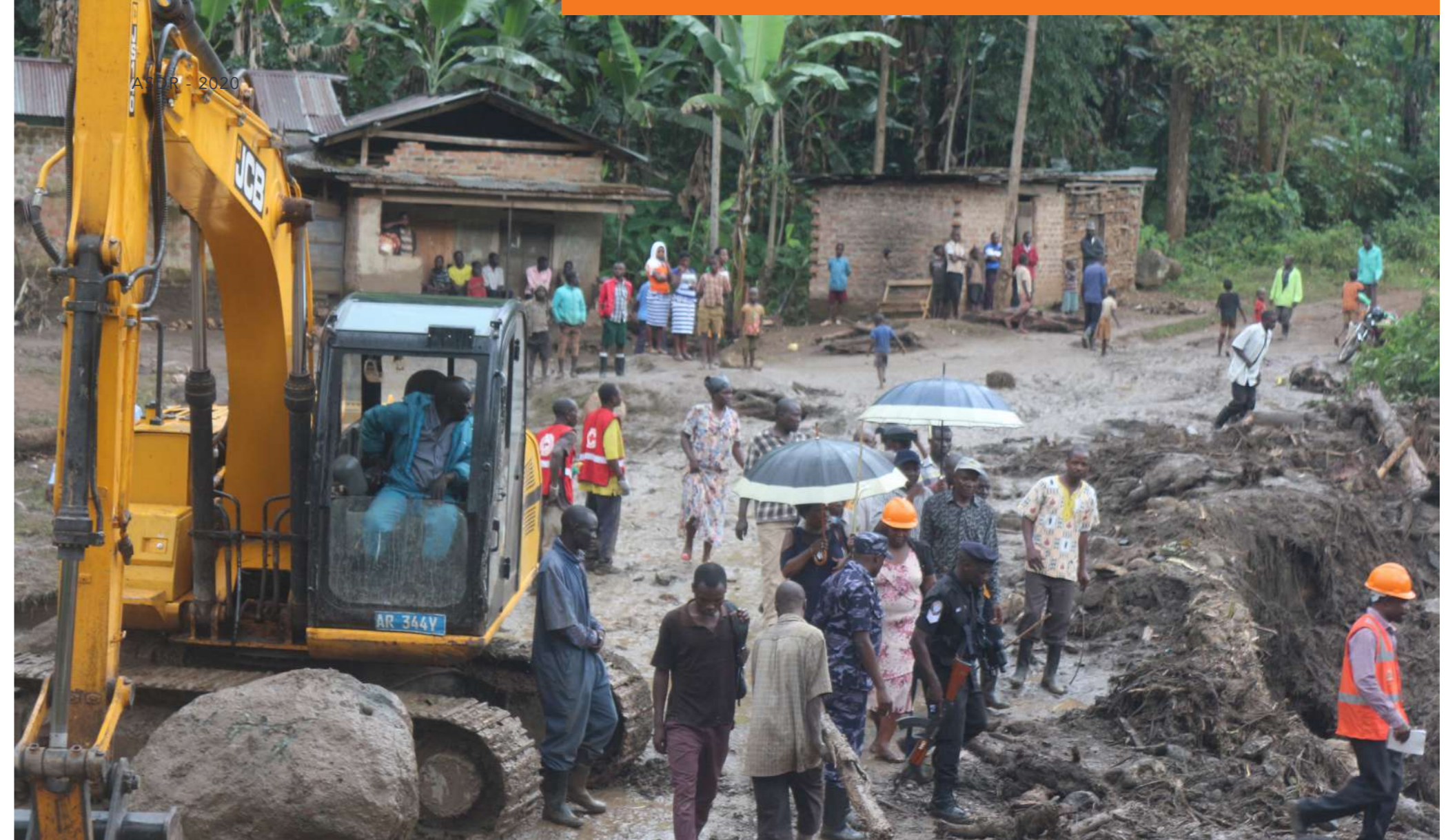
A section of Bukalasi Road, Bududa District damaged by landslides being reopened using Local Government works equipment.
